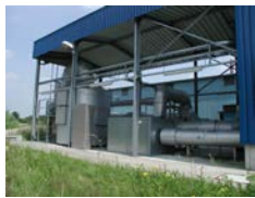
Catalytic oxidation (KNV), 11.000 Nm 3 /h
