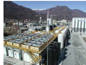
Ground water treatment plant, 850 m 3 /h
