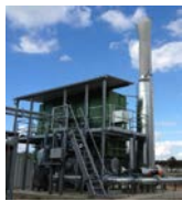
Regenerative oxidation (RNV), 3.300 Nm 3 /h
