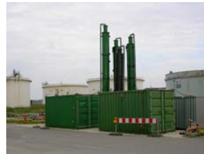
Batch treatment plant for process waste water treatment
