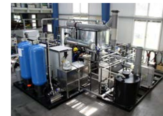
Regenerative activated carbon filter solvent recovery
